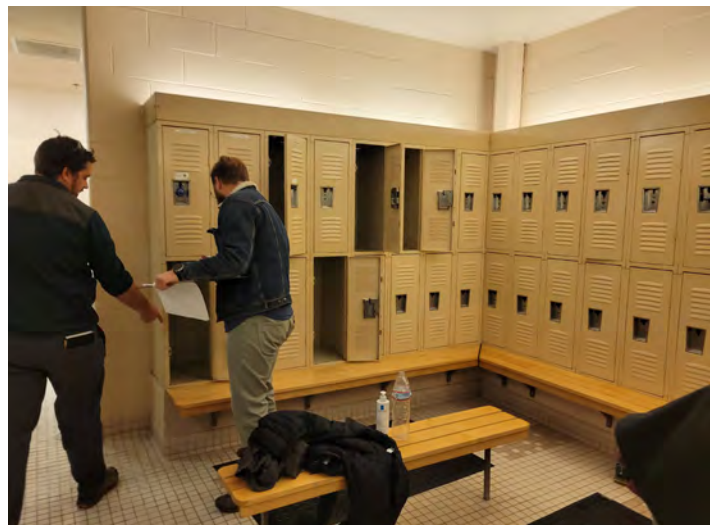
6. EPRD staff showing rust and damage to BRS
