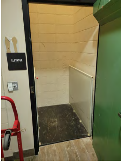
1. Lift only serves 1st and 2nd floor, 3rd floor not accessible
