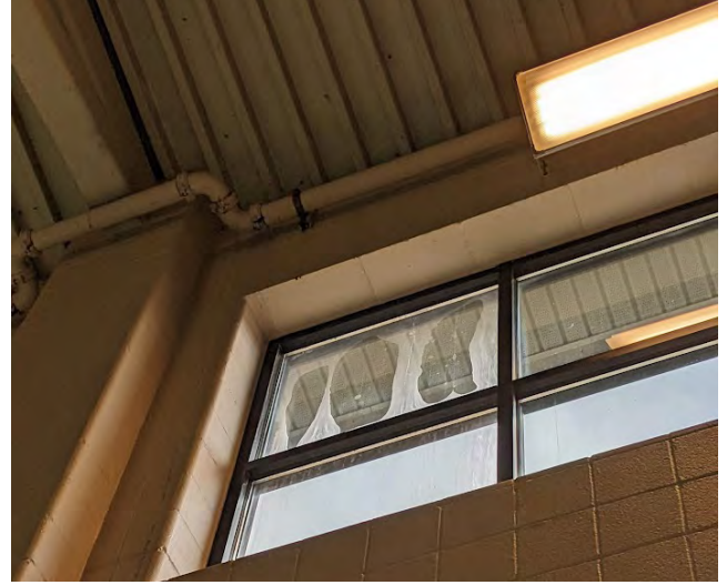
2. Damaged glazing in pool
