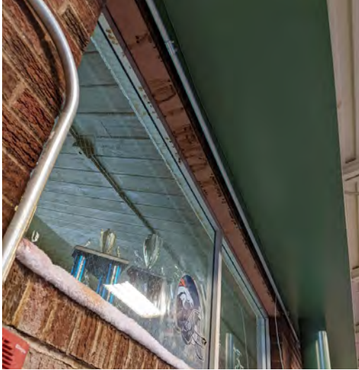
7. Staining from leak, towel to catch condensation
