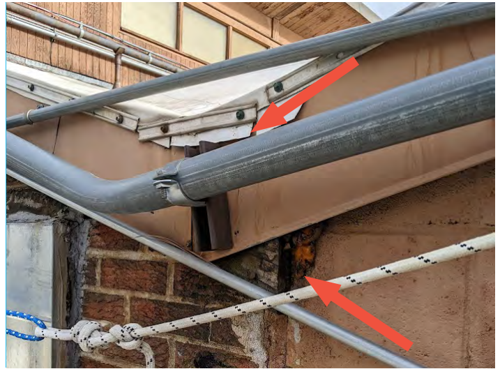
4. Gaps in building and flashing damage
