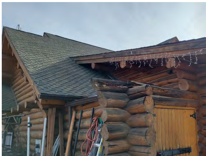
4. Damage to upper logs
