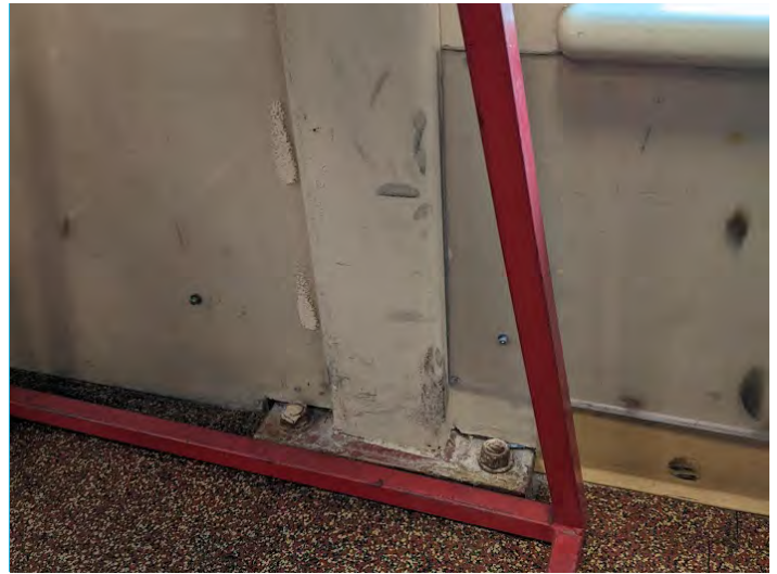
4. Acrylic panels to prevent further damage
