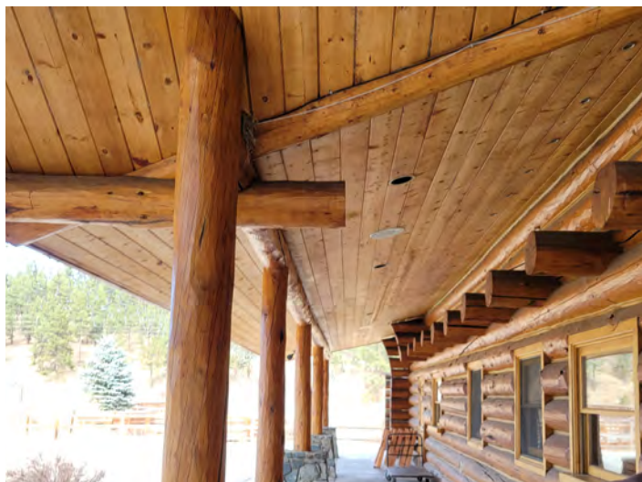
3. Leaks occurs in office space with windows at right
