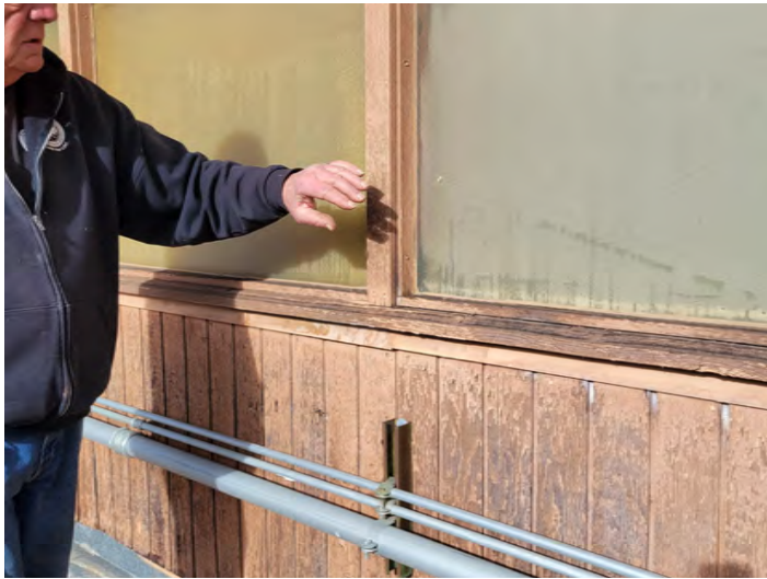
3. Leaks and damage at wood siding & windows
