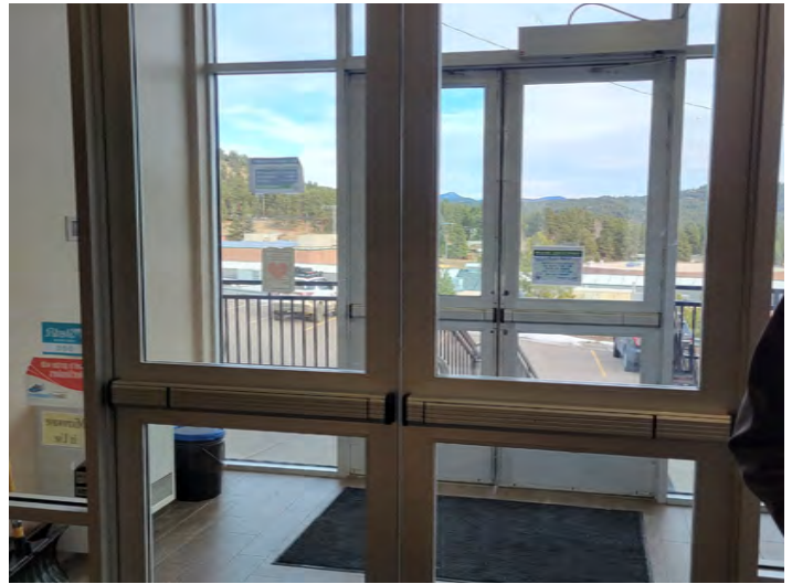
10. Front exterior entry doors to replace with auto sliders
