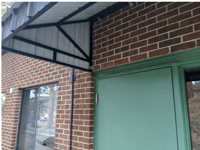
5. Flashing missing at exterior doors & windows
