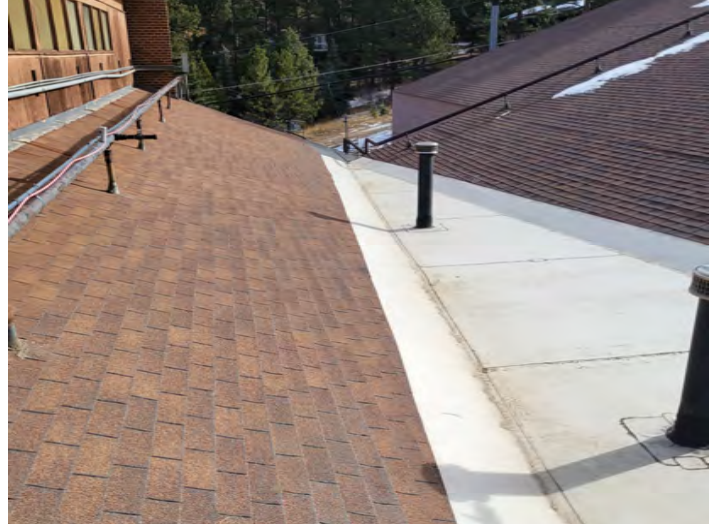
2. Asphalt and membrane roof leak
