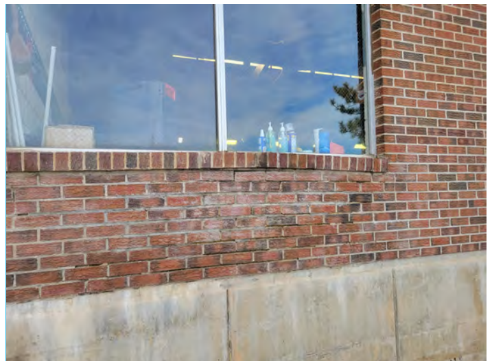
6. Damage at exterior wall & window
